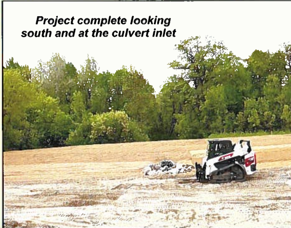
During construction Picture Shaping the Earthen Berm and Grassed Waterway - Looking East
